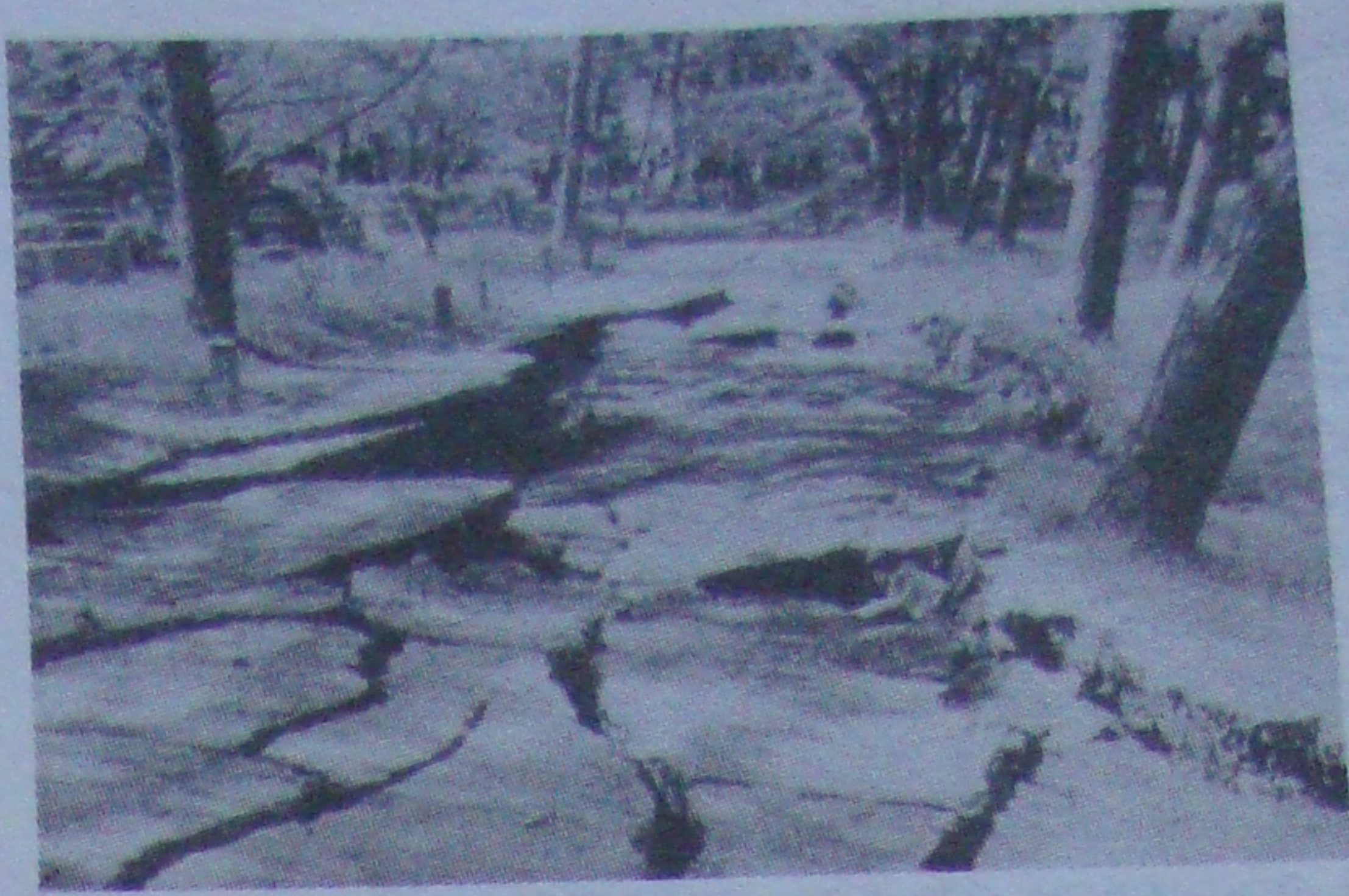
Photo 2 Cracks in the road leading to the graveyard in Aoba-cho
